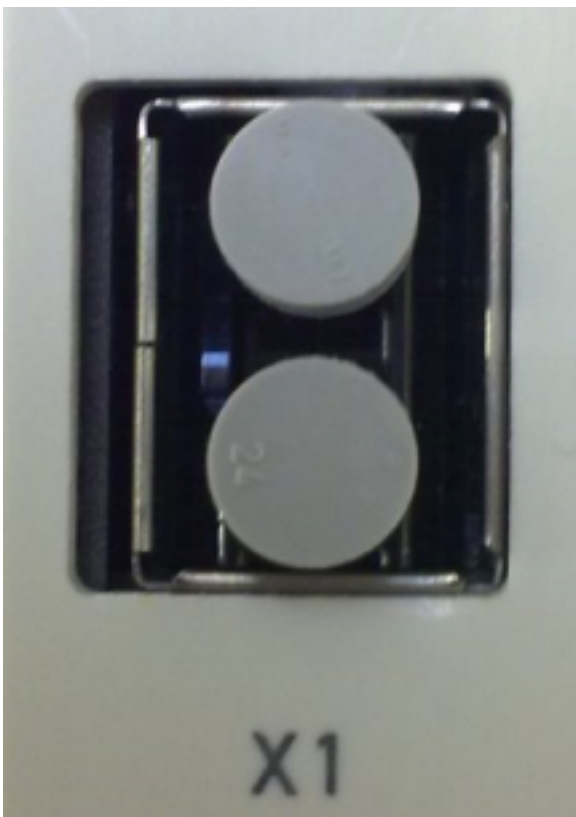
Figure: Blind plugs in unused sockets
