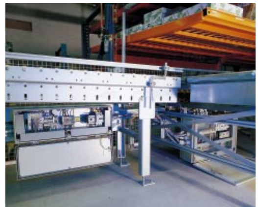
One switching cabinet is responsible for each transport unit. An advantage of this solution is high flexibility when remodelling the plant. In order to release a circuit module, and thereby the transport module, only six cables have to be disconnected.
